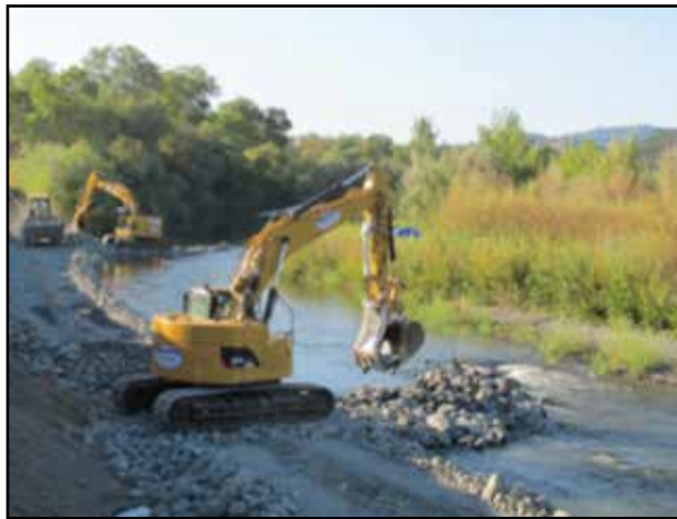
The LST was made wider to provide a ‘feeder’ access for rock.
