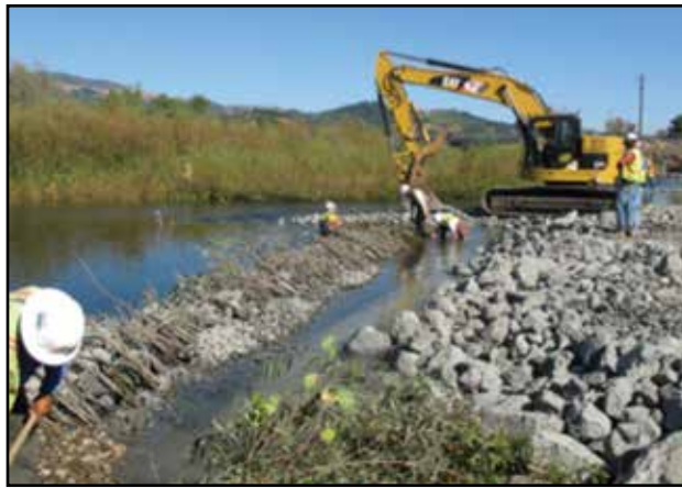
Live Siltation installed deeply in trench - self-filtering rock used to control turbidity.
