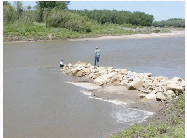
Figure 2. A stone bendway weir, an example of a redirective bank protection technique.
