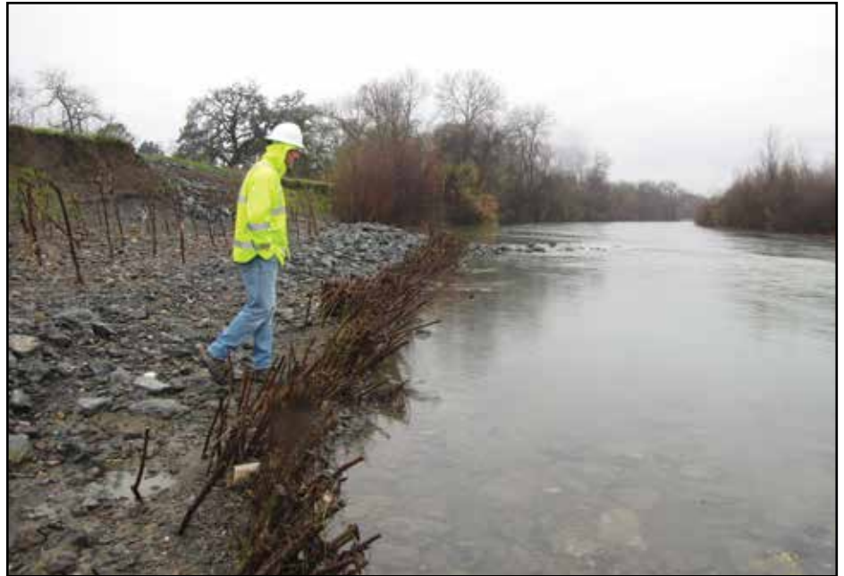
The Russian River project after high flows recede. Note the rock, the live siltation and the pole plantings are still in place. January 13, 2011
