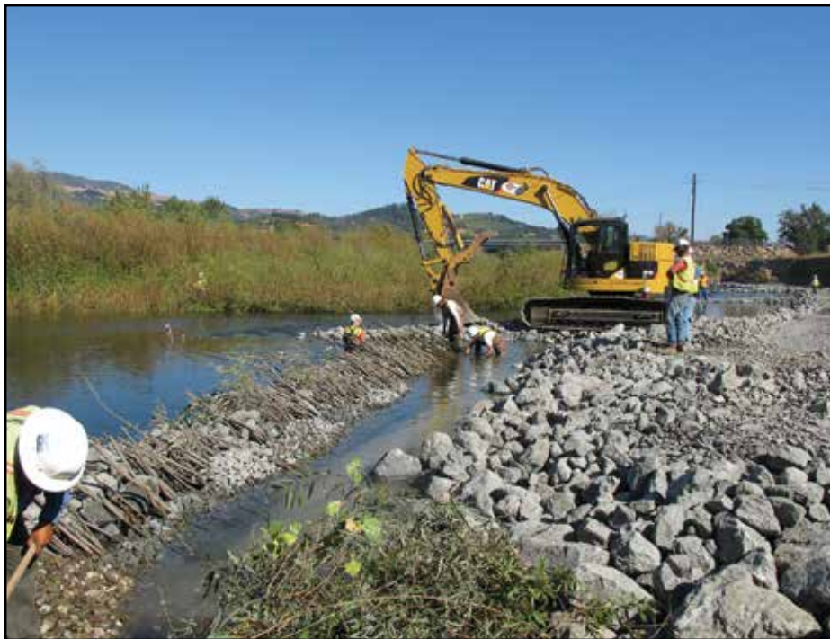
Geyserville Bridge project installing Live Siltation behind LST. Note how the self-filtering gradations minimize turbidity.
